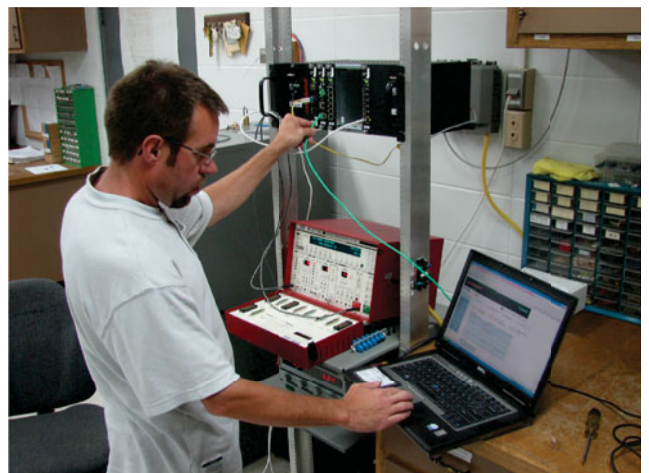
NIPCO Technicians only require a laptop to perform JumboSwitch network health/alarm checks and reconfigurations.
