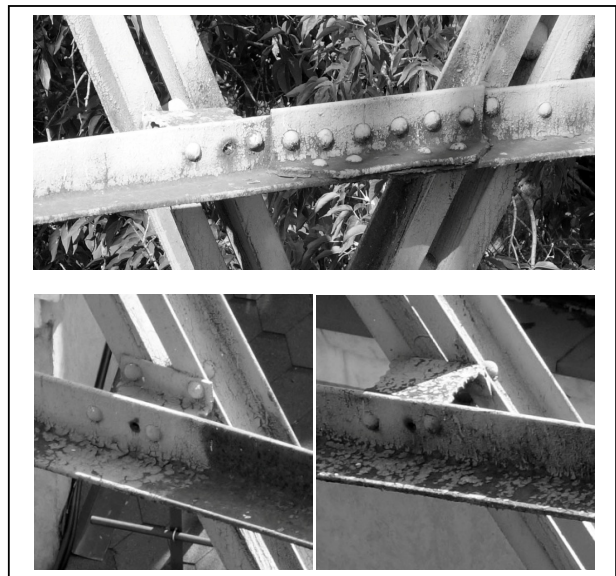
Fig. 4. Unused holes in the 3rd intermediate ring of the 1st section.
